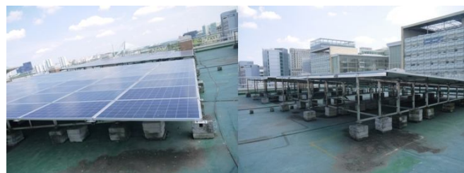
Figure 3: Existing Solar PV Panels at LAS building
