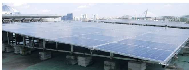
Figure 2: The installed PV Panels at LAS building
