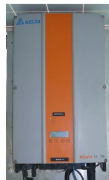
Figure 4: The existing inverter
