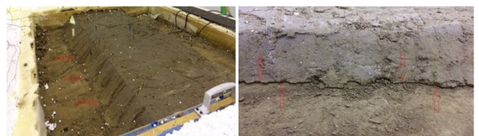
Figure 6: Detachment of the sloping part of the sub-grade from the road base.
