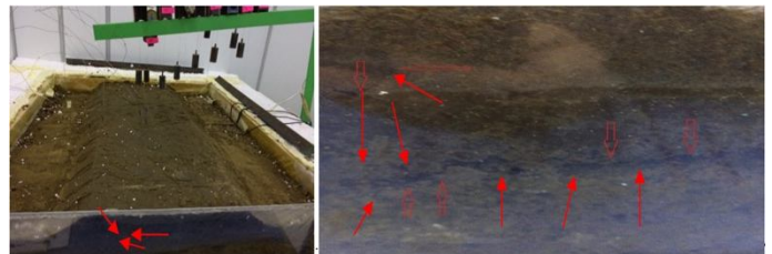
Figure 5: A crack in the body of a roadbed embankment.
