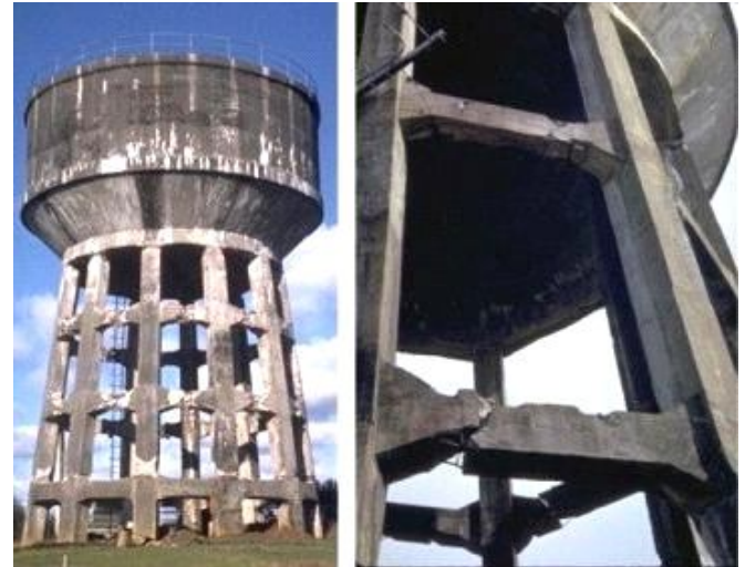
Fig 1.1 Failure of braces because of earthquake
