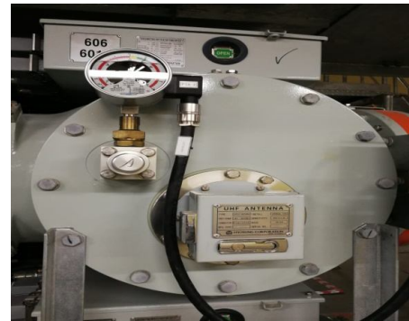
Figure 6: UHF Sensor installed on GIS
