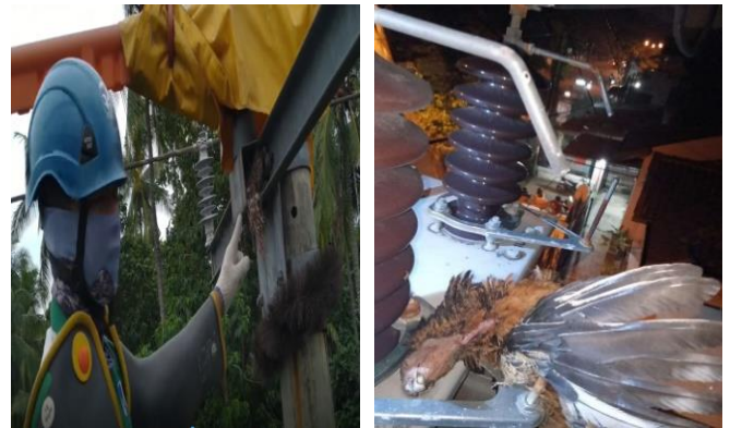
Figure 8: Bird nest and some bird corpses were found in the transformer mechanics.
