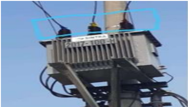
Figure 12: Bird barrier on the bushing transformer.
