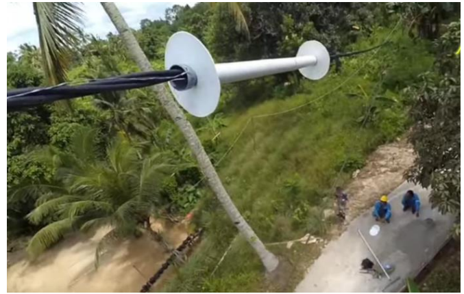
Figure 15: several animal crawling barrier (2).
