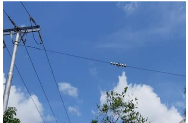
Figure 9: Bird barrier block is installed on the transmission line.
