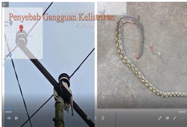
Figure 6: Snakes interferences into the transmission lines.
