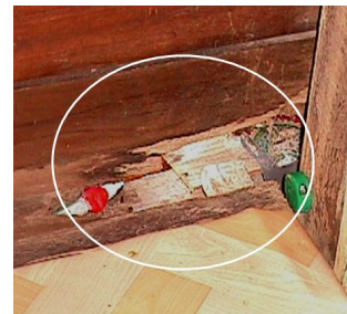
Figure 12(b): Rotted wallboard
