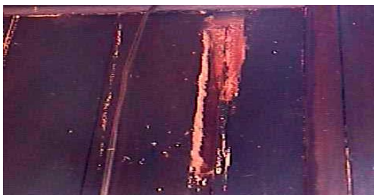
Figure 19(b): Rotted wall
