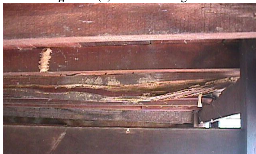
Figure 28(b): Rotted floor girders
