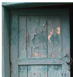
Figure 22(a): Peeling paint
