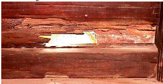
Figure 19(a): Decayed wall
