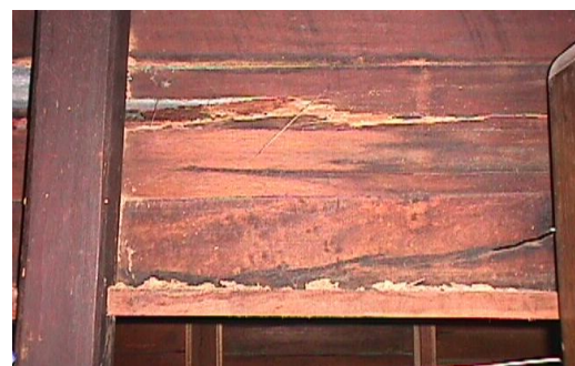
Figure 29(b): Rotted wallboard
