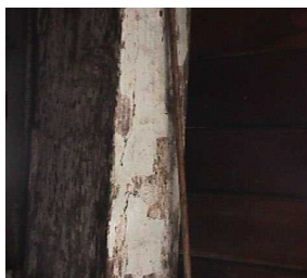
Figure 3(a): Rotted pillar
