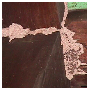
Figure 21(c): Rotted roof beam
