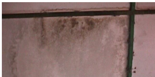
Figure 25(d): Dirty ceiling surface
