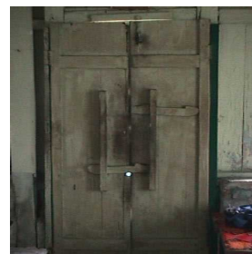
Figure 5(a): Dirty door
