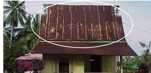
Figure 16(a): Rusted zinc roof finishes
