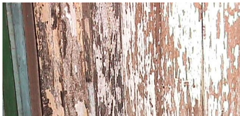
Figure 2(d): Peeling paint finishes
