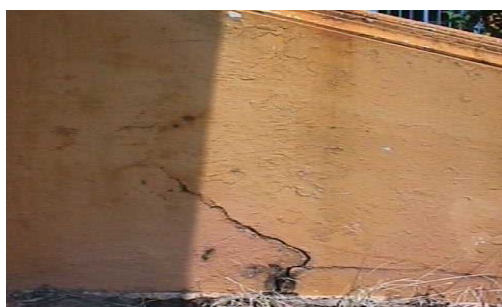
Figure 26(a): Cracked stairs
