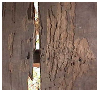
Figure 10(a): Rotted boards
