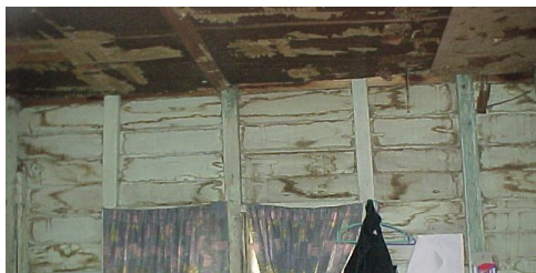
Figure 2(c): Dirty stains on walls
