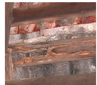
Figure 16(f): Rotted beam
