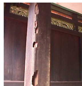
Figure 20(a): Rotted pillar
