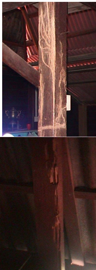
Figure 30(a): Decayed pillar
