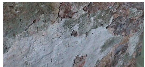
Figure 6(a): Falling off plaster
