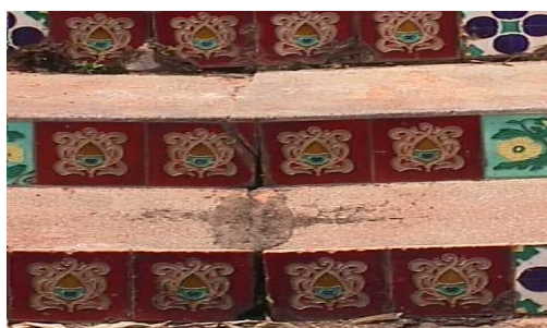
Figure 26(b): Cracked steps
