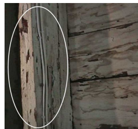
Figure 3(b): Rotted pillar
