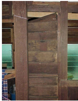
Figure 29(d): Fallen wall
