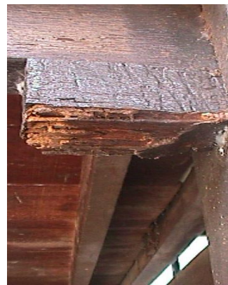
Figure 31(a): Decayed crossbeam
