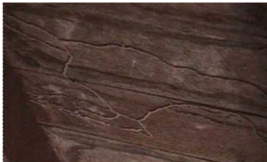
Figure 18(b): Rotted floor boards
