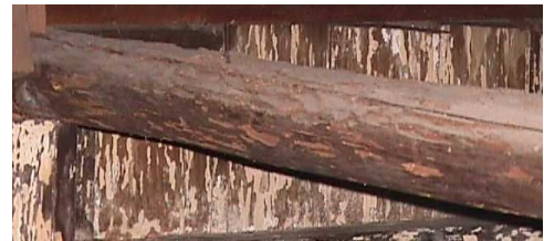
Figure 4(a): Decayed roof crossbeam
