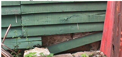
Figure 2(b): Falling off wallboard
