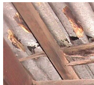
Figure 16(e): Holes on roof
