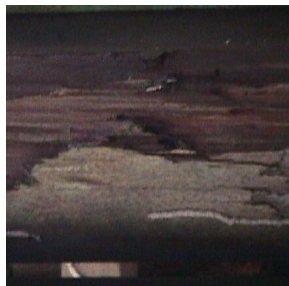
Figure 21(d): Rotted roof beam
