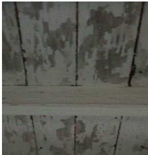
Figure 7(a): Peeling paint
