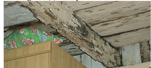
Figure 4(b): Rotted floor crossbeam
