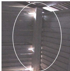
Figure 12(a): Rotted wall
