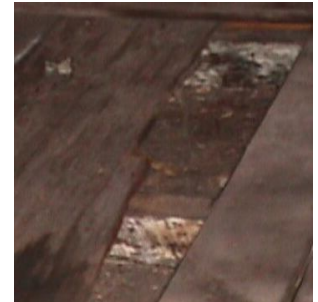
Figure 1(b): Detached boards
