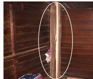
Figure 13(b): Decayed pillar
