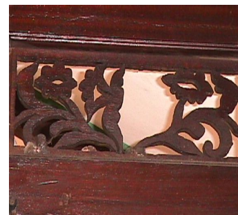
Figure 24(b): Broken fretwork
