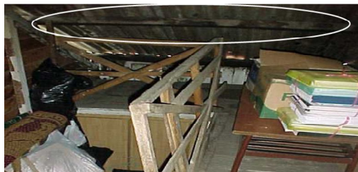
Figure 8: Dirty stains on roof rafter
