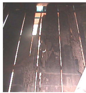
Figure 28(c): Rotted floor
