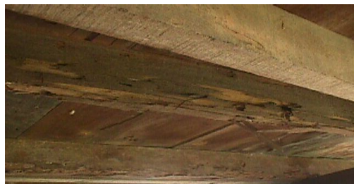
Figure 28(a): Rotted floor girders
