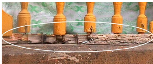
Figure 15(b): Rotted window frame
