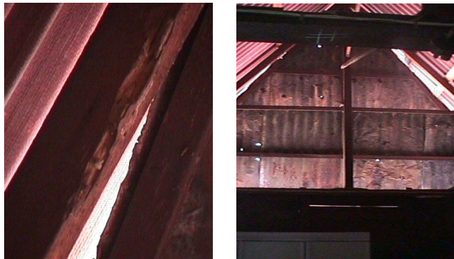
Figure 34(a): Rotted rafter Figure 34(b): Rusted “tebar layar”
