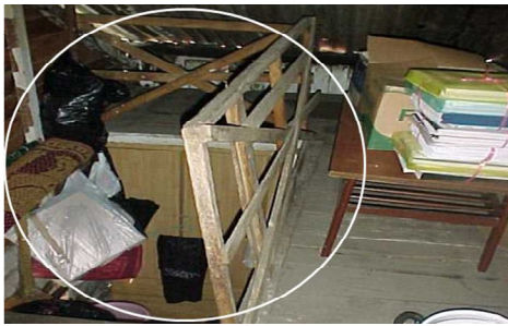
Figure 6(b): Unstable wood staircase and handrails
