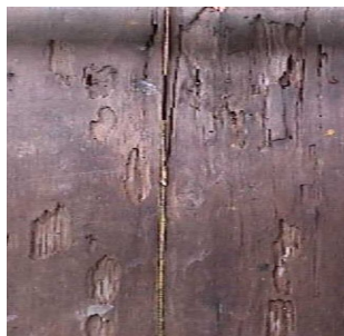
Figure 10(b): Rotted floor
