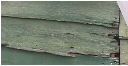
Figure 2(a): Rotted wallboard
