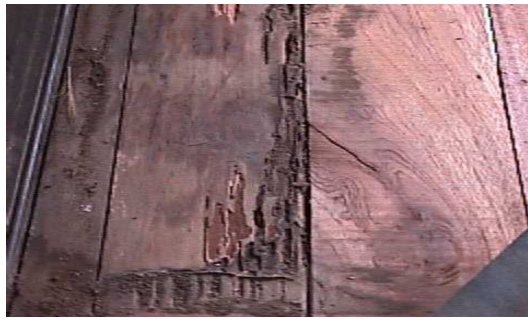
Figure 18(a): Rotted floor boards
