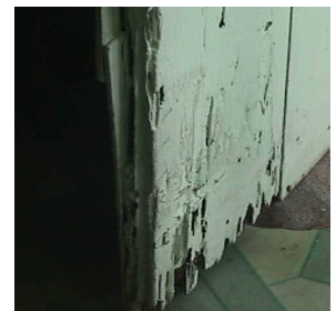
Figure 5(b): Decayed door
