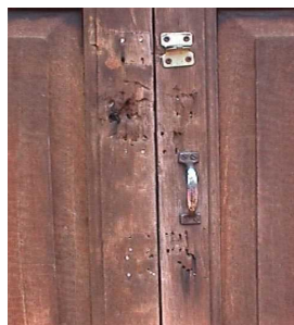
Figure 22(b): Broken surface
