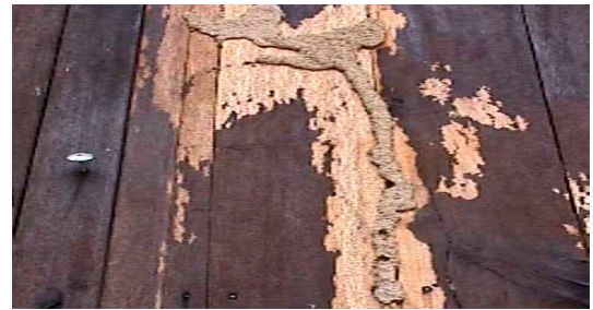
Figure 19(c): Pest nests on timber wall
