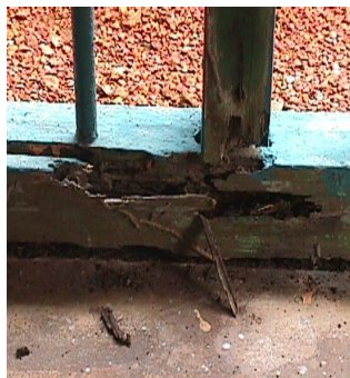
Figure 23(b): Rotted frame
