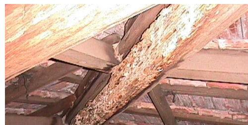
Figure 25(c): Decayed roof rafter
