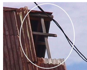
Figure 16(b): Fallen finishes
