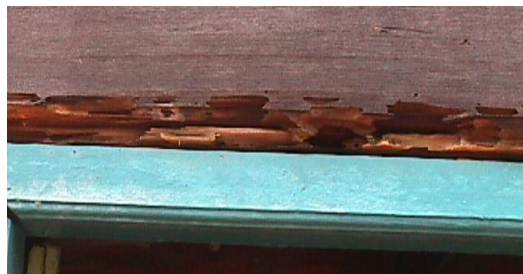
Figure 21(b): Decayed floor crossbeam
