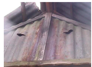
Figure 16(c): Rusted “tebar layar”
