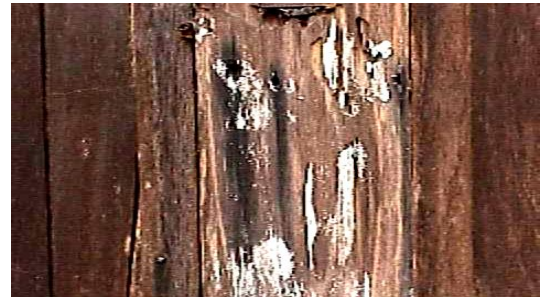
Figure 19(d): Deteriorated wall
