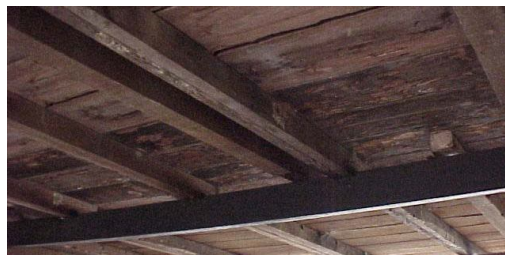
Figure 10(d): Decayed joists and floor boards
