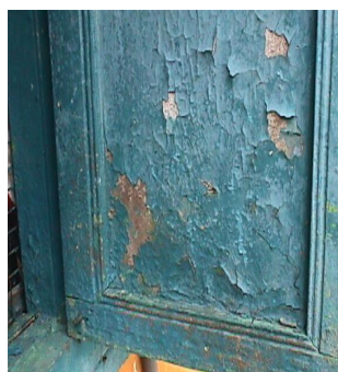
Figure 23(a): Peeling paint
