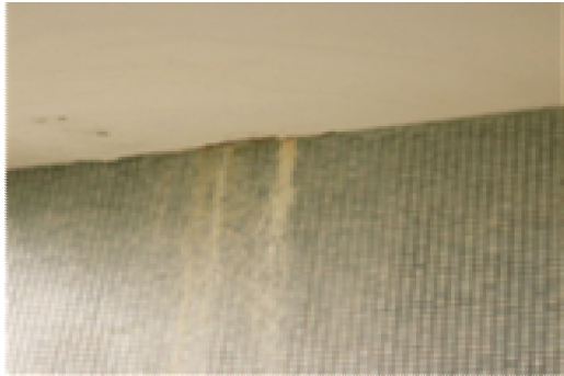
Figure 36: The possible fungus colony here at the mosaic wall is created from the water seepage from the edge of the floor and concrete wall as found at this academic building.
