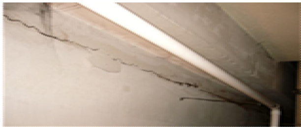
Figure 21: This concrete beam running through-out the toilet showing its detachment process in the making due to water leakage from the top wet area.
