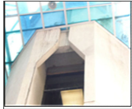
Figure 4: Dampness being created from the expired sealant of the skylight and can be tracked from the stained wall of this interior of an office building
