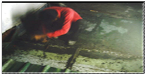
Figure 8: A rare view of the internal part of an enclosed space having the water ponding effect letting seepage to the public interior space below
