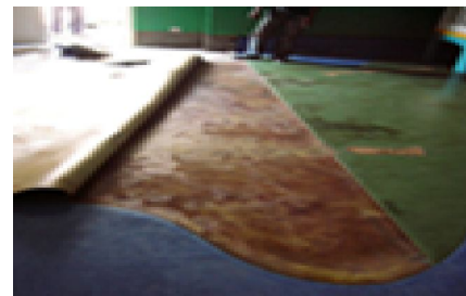
Figure 19: Closure look on the linoleum flooring found at this hospital's children playground detaching itself due to water seepage
