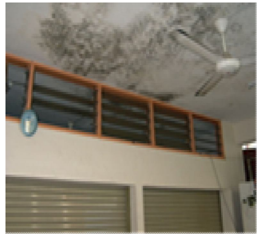
Figure 38: The formation of hazard like condition may let fungus to grow even on top of the paint layers of these concrete floor slabs. The interior become unhealthy due to tiny particle trapped inside the room
