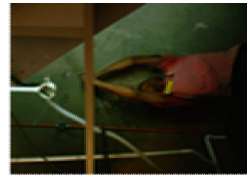
Figure 17: (right) show a typical stained appears once you removed the stained ceiling tile.
