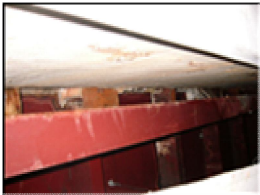
Figure 37: The formation of hazard like condition may let fungus to grow even on top of the paint layers of these concrete floor slabs. The interior become unhealthy due to tiny particle trapped inside the room
