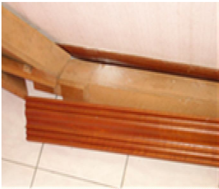
Figure 32: Wear and tear of the timber skirting and parquet floor with the help of the humidity of the internal space creating this mess
