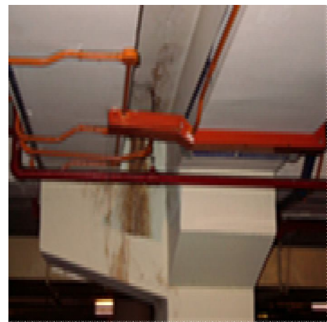
Figure 39: These are another example of the hazardous fungus effects particles found within the interior space of this leakage concrete. This defect found within the internal part of the parking basement area and getting worse affecting the parked cars
