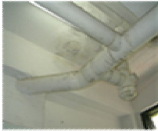
Figure 12: Typical problem due to the under slab concrete leakage with clear stained marked on it possible due to building movement.
