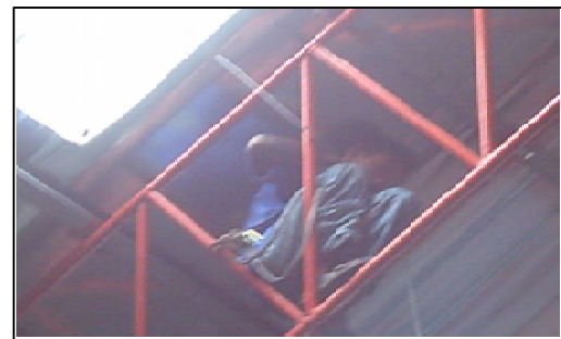
Figure 30: The maintenance crew squeezing himself in making rectification work repairing the hole using the fiber mat and antirust paint for this internal part of the metal roof material.
