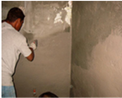
Figure 41: Anti-fungus coating is being applied for this rectification work of an interior space. The task requires expert personnel to ensure the space back to its original condition and in reusable state
