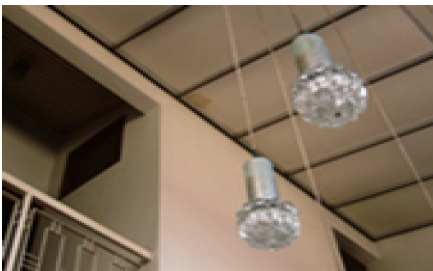
Figure 3: Defect found with stained ceiling tile at this double height space with elaborate lighting invites problem
