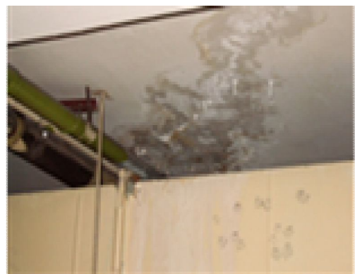
Figure 40: These are another example of the hazardous fungus effects particles found within the interior space of this leakage concrete. This defect found within the internal part of the parking basement area and getting worse affecting the parked cars.
