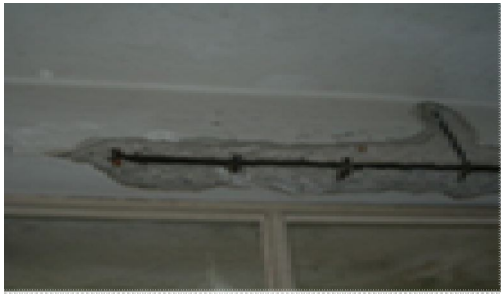
Figure 20: Structural repair required for this concrete spalling task due to detachment defects found at this internal part of the room
