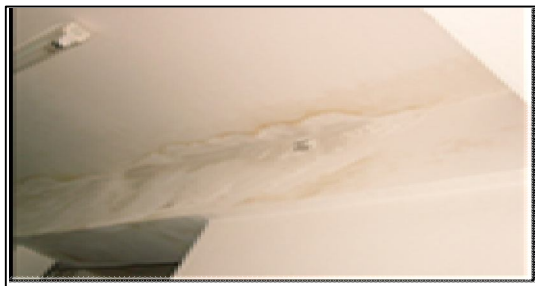
Figure 2: The dampness effects clearly be seen at this beam due to minor leakage from the above wet area
