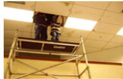
Figure 5: Workers checking the dampness space between the ceiling interior and the underneath concrete slab
