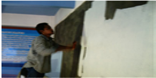
Figure 1: Interior dampness rectification work been treated for this museum interior been treated by maintenance crew
