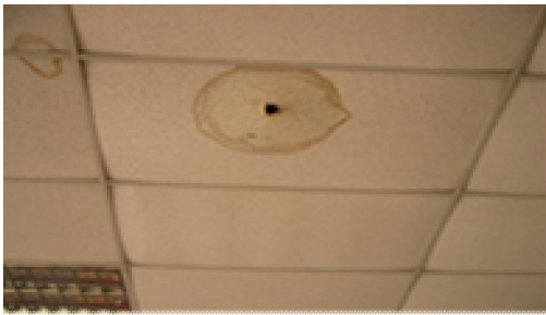
Figure 35: Possible fungus formation seen at this ceiling tile may hazard the occupant of this space and also can become an ideal breeding space for termites to make a colony.
