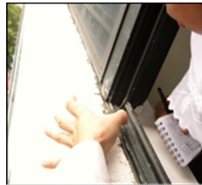
Figure 29: Wear and tear usage for the expired window sealant found at an office building
