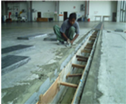
Figure 26: The wear and tear of the floor material pays its toll due to the heavy vehicle load as well due to frequent traffic usage at airport hangar building
