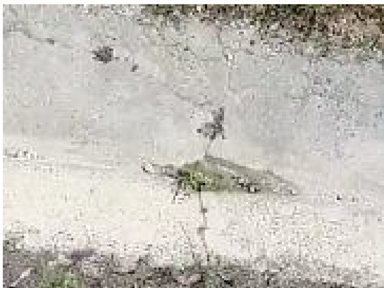
Figure 14: Zoom Image for Crack at Height 9 Meters
