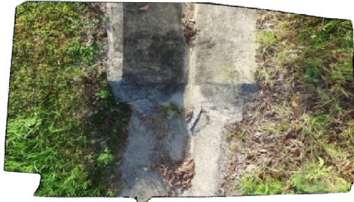
Figure 9: Damage Analysis of 3D models Crack No 1
