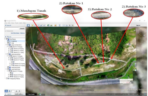
Figure 12: Damage position at The Slope Structure in Google Earth Pro
