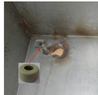
Figure 10: Insulator bushing gone
