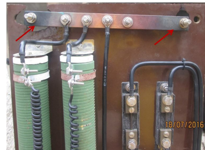
Figure 4: Heating sign on copper busbar
