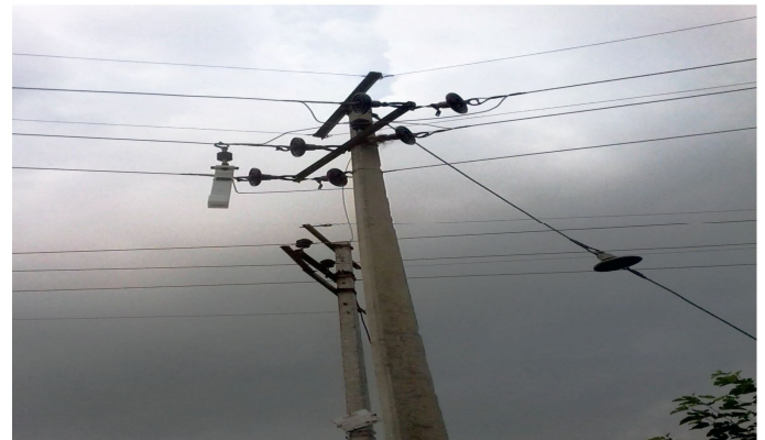
Figure 3: Field test conducted at the pole
