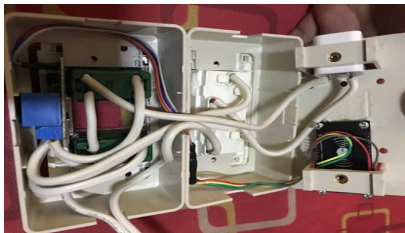
Figure 7: Casing and Components inside the Modular Box
