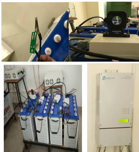
Figure 6: Battery with BMS devices and Inverter system
