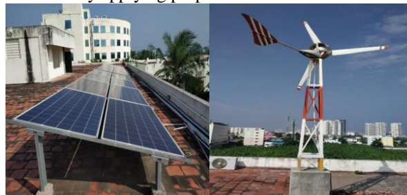
Figure 3: Solar Panel 5KW installed in the Campus and 1KW Wind Mill PMSG installed
