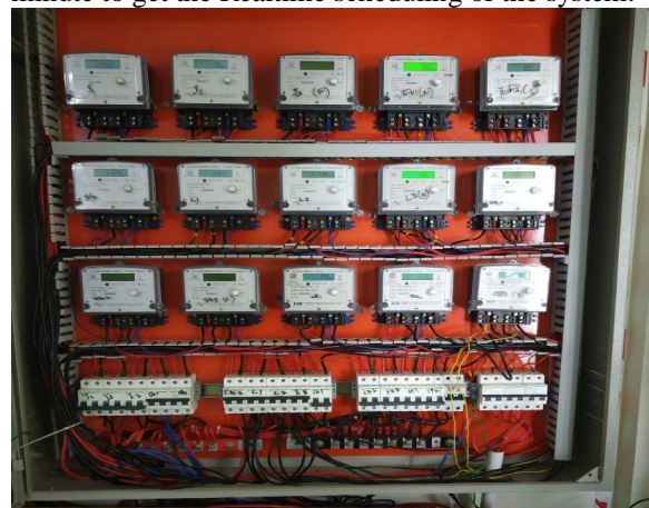
Figure 7: Master controller of EMS with MCB and BUSBAR AC for Sharing and Controlling
