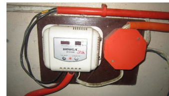
Figure 4: Charge Controller (PWM) replaced with MPPT.
