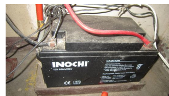
Figure 5: Storage Battery (Lead Acid Battery)
