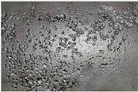
Figure 3: An example of general deep pitting corrosion with some pits joining to form larger pits and interconnected pitting.
