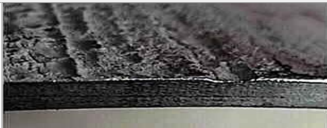
A cross sectional view of corrosion and cracking. This profile illustrates that when the combined depth of the corrosion and cracking is considered a significant percentage of the total wall thickness may be lost.
