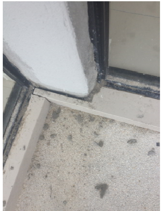
Figure 6: Gaps between floor base and column
