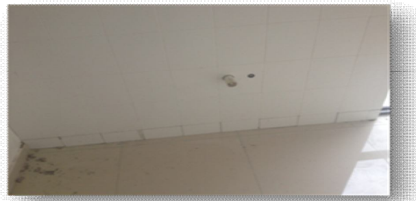
Figure 5: Uneven tile lining
