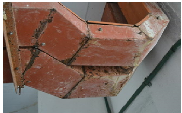
Figure 3: Corrosion on external metal trunking
