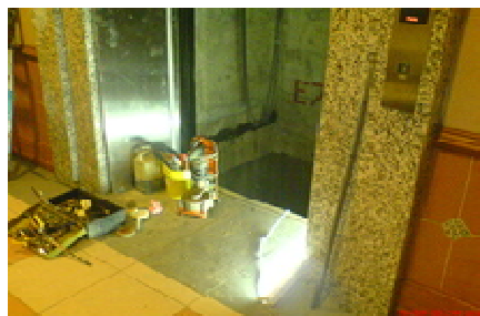
Figure 19: External view of the lift pit- to be closed for rectification work
