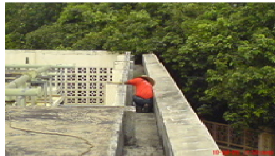
Figure 15: Clogging off concrete gutter
