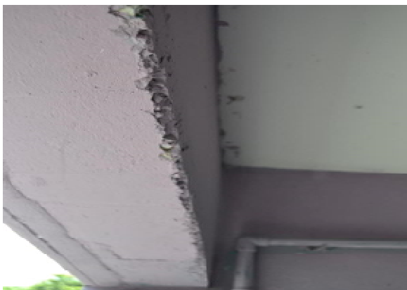
Figure 2: Honeycombing defect problem
