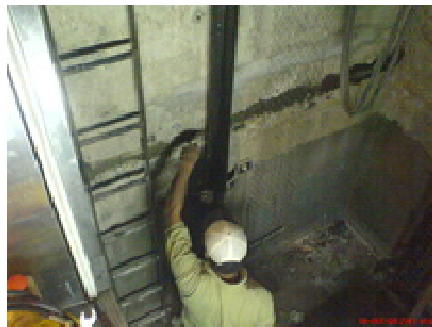
Figure 18: Water seepage at the lift pit wall due to high water table
