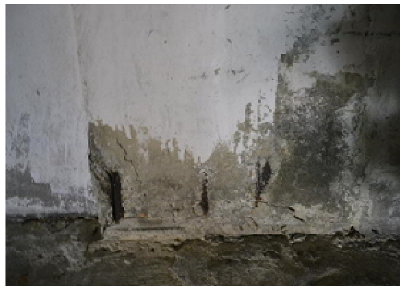
Figure 1: Concrete surface damage
