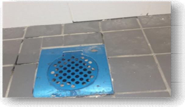
Figure 4: Tiles grouting improper
